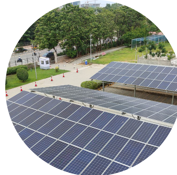
Images: Solar panel installations in parking areas of our Hyderabad campuses
